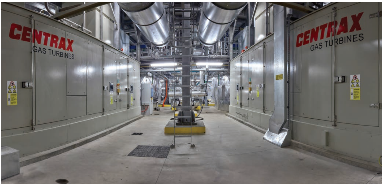
Photo credit: Centrax Gas Turbines
