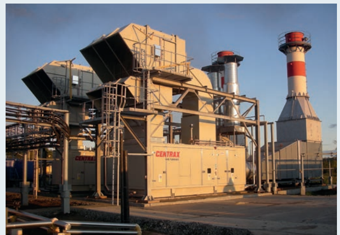
Photo credit: Centrax Gas Turbines
